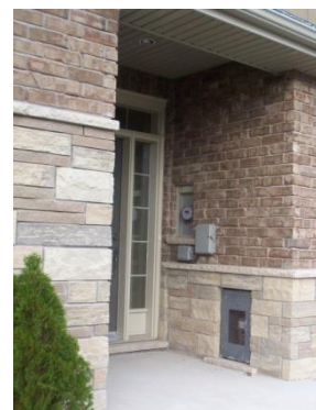
Example of Recessed Utility Meters on Townhouses
